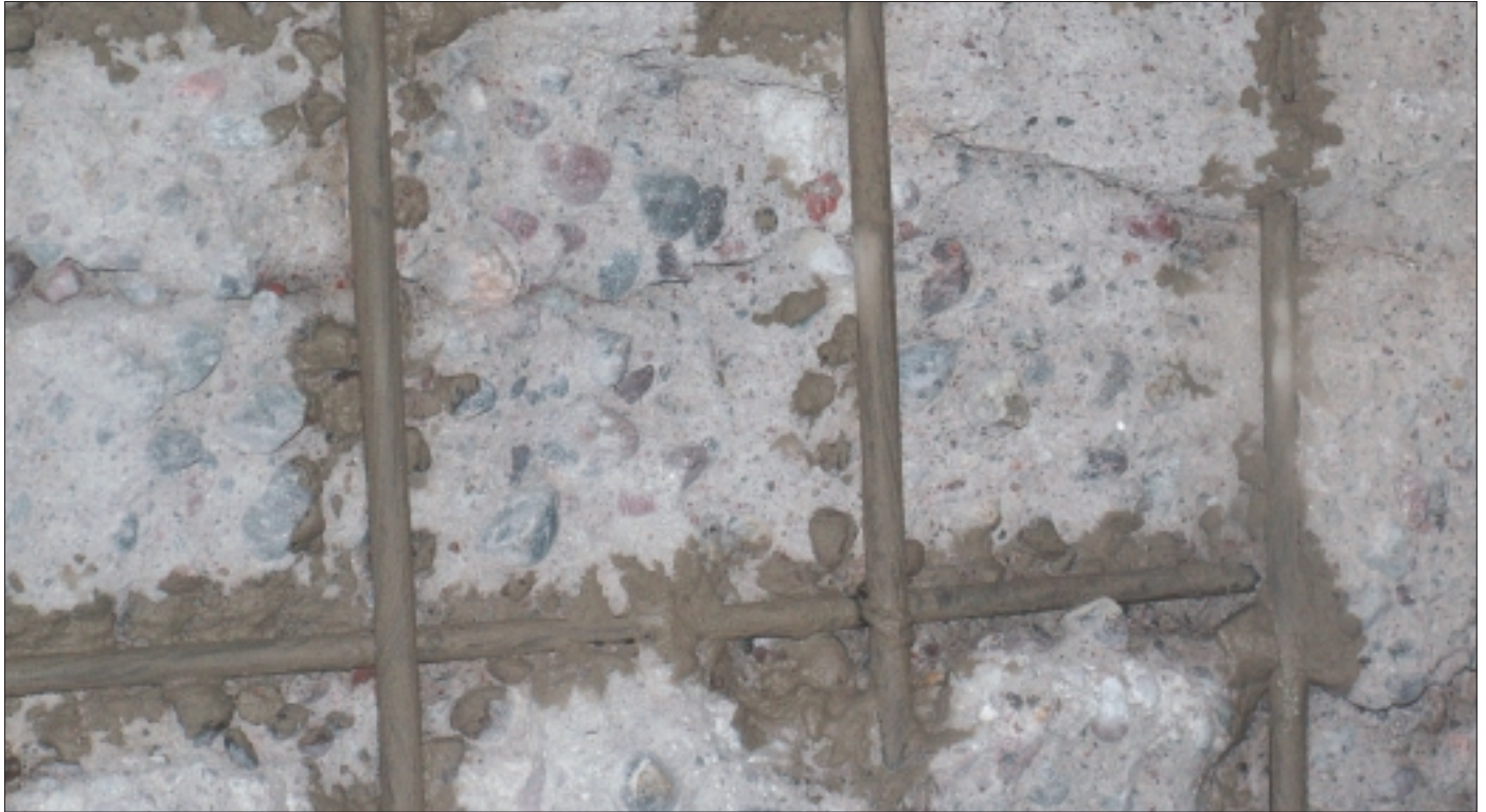
The walls of the tunnel, were cleaned from carbonated concrete by the water jet method, the reinforcement bars were protected before a new surface was built with high performance polymer concrete. The last stage to protect the concrete from moisture, was to crystallise.
